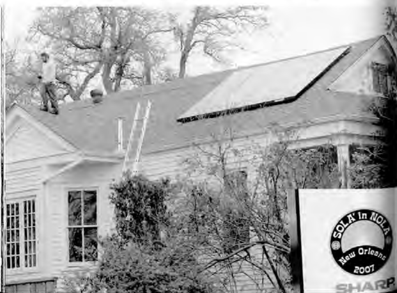
Figure 30.13 (Below) House on Jourdan Street, Lower Ninth Ward, retrofitted with solar panels. One of ten installations by Sharp Corporation's 'Sola' in 'NOLA' initiative, supported by the Preservation Resource Center and the Louisiana Department of Natural Resources. (enerG Magazine)
